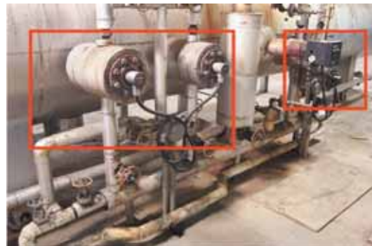
ORIGINAL FLOAT SWITCH INSTALLATION
