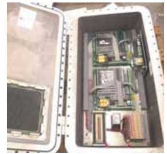
LEVEL ELECTRONICS WITH ZENER BARRIERS
