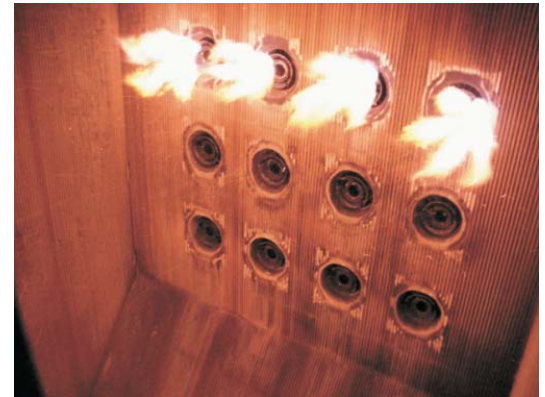
OIL IGNITOR FLAMES
